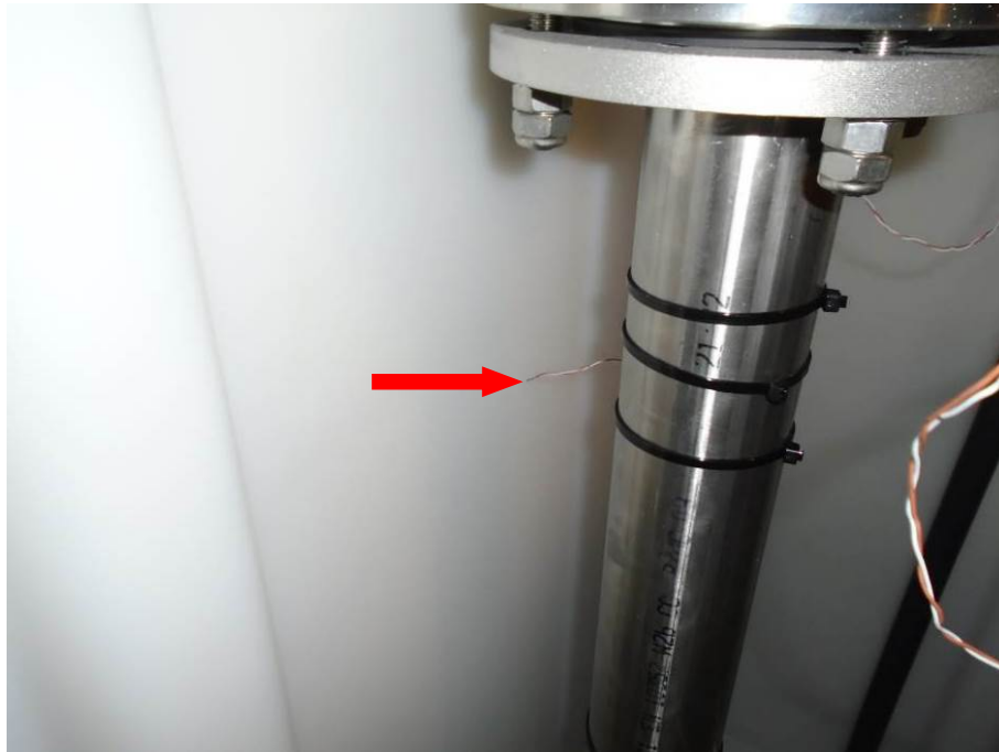
Figure 2.1.3 Middle thermocouple (pre-installed by Hughes Safety Showers Ltd)
