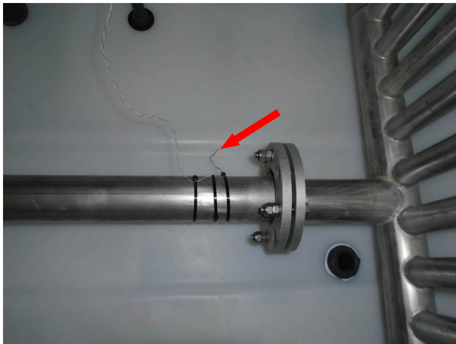
Figure 2.1.4 Bottom thermocouple (pre-installed by Hughes Safety Showers Ltd)
