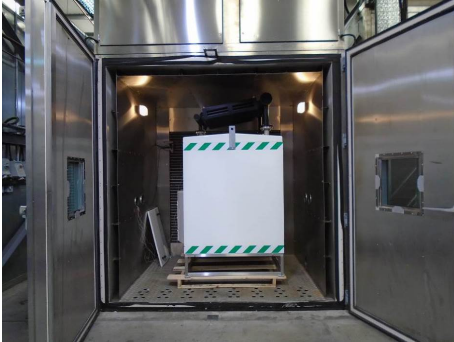
Figure 2.1.1 Passively cooled emergency tank shower located in walk-in chamber
